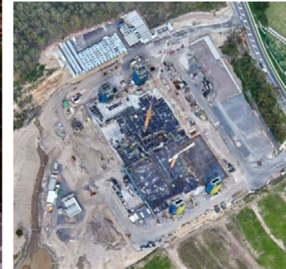
New Maitland Hospital Development \ A substantial civil works package was required to ensure site access, roads and parking and drainage from the site.
